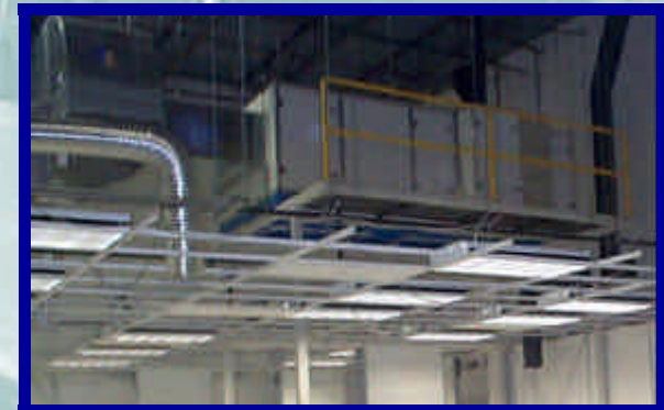
Stand Mounted Air Handling Unit
