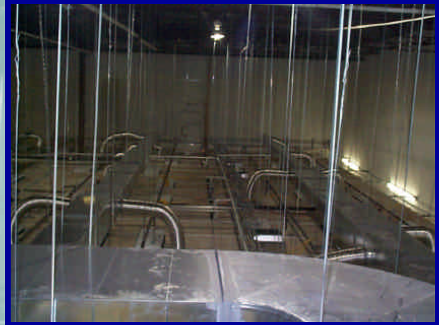
Supply Air Ductwork to HEPA Filters
