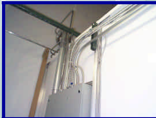
Electrical Panel Rear View
