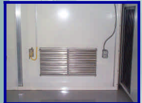
Return Air Grille Electrical & Data
