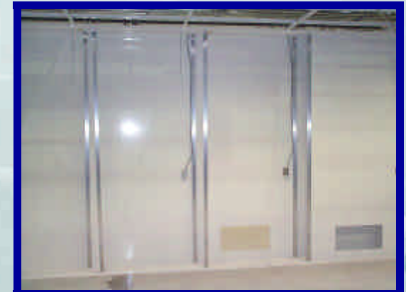
Double Wall for Return Air
